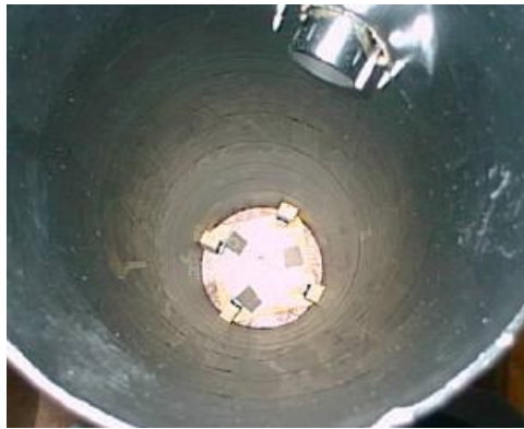
Figure 12: The installed tailgate, viewed from down the tube. You can see the mounting blocks holding it in place.
